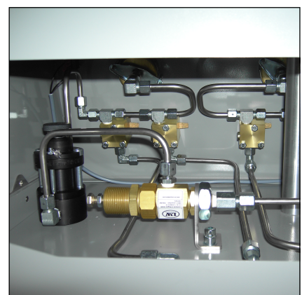
Fig. Safety valve on the left: 225 bar, pressure reducer on the right: 330 / 225 bar
