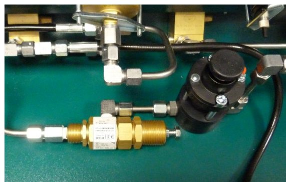
Fig. (left) Pressure reducer; (right) safety valve
