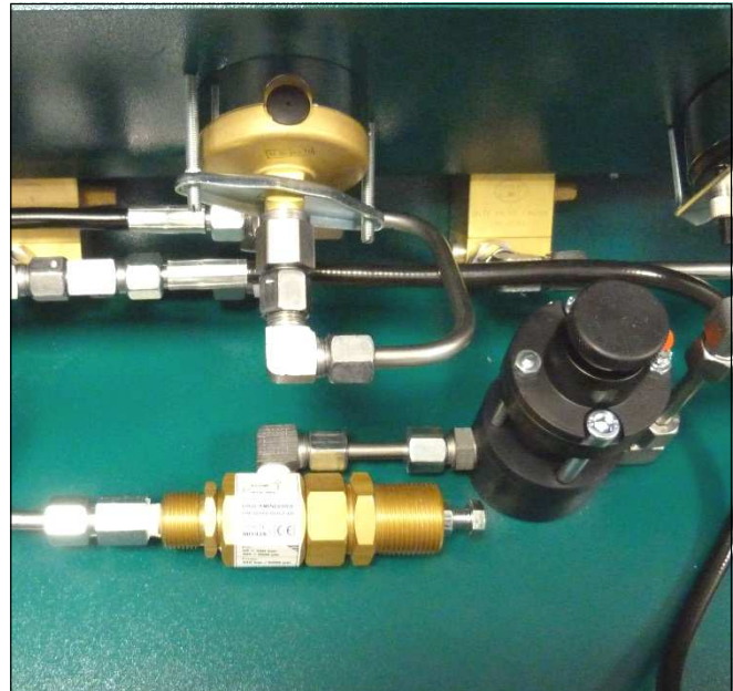
Pressure reducer (left) & safety valve (right)
